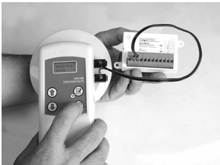
Figure 35 - Addressing modules using a VPU100
